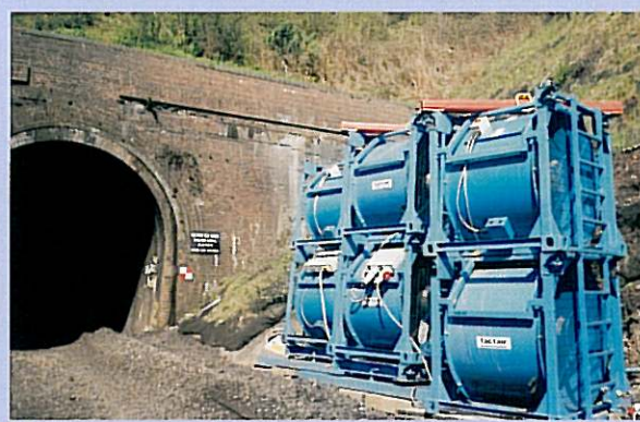
Ventilation Fans Deployed at Patchway Tunnel
