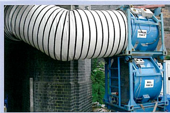
1200mm Diameter Electric Powered Fans
