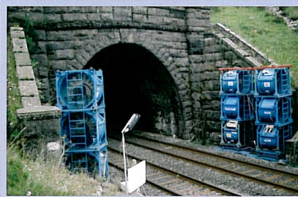
Ventilation Fans Deployed at Bleamoor Tunnel
