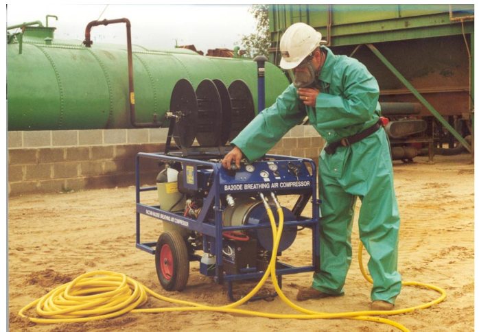
Final checks on a BA20DE mobile breathing air compressor prior to entering an oil storage tank.
