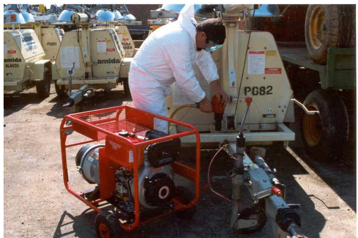
An engine driven unit being used to repair a mobile lighting tower.
