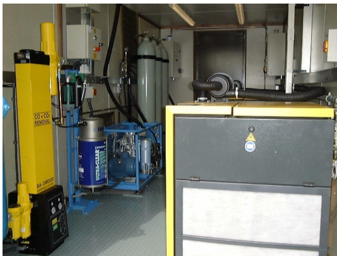
Automated breathing air system
