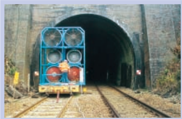
Trailer Mounted Ventilation Fans Deployed at Foxhill Tunnel
