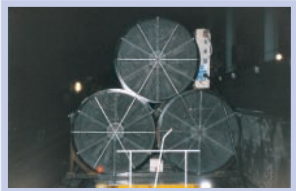
1000mm Diameter Fans In Sub-Surface Railway Tunnel
