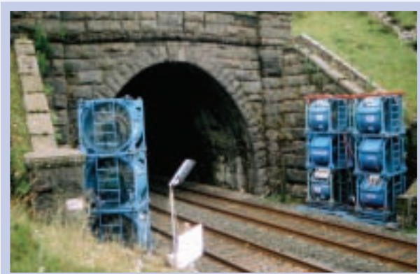
Ventilation Fans Deployed at Bleamoor Tunnel
