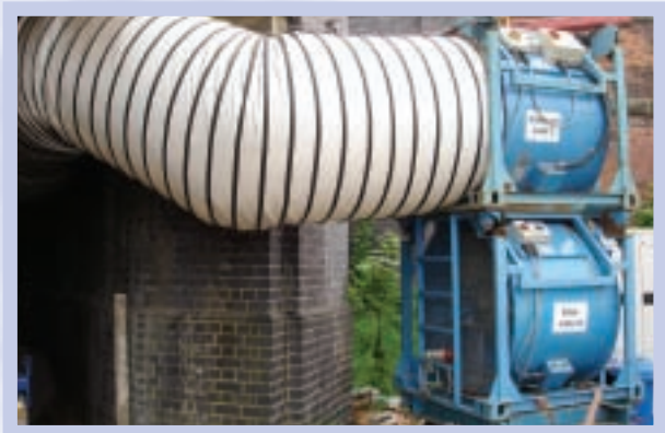
1200mm Diameter Electric Powered Fans
